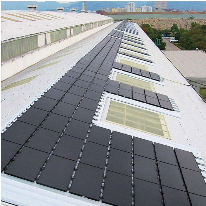
▲ CIS thin-film photovoltaic panels on the Kokura Factory rooftop
