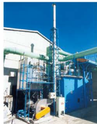
Waste Gas Condensing and Oxidizing System 浓缩废气处理系统
