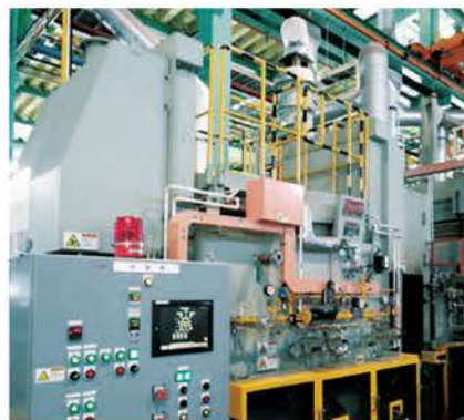
Continuous Gas Soft Nitriding Furnace 连续气体软氮化炉
