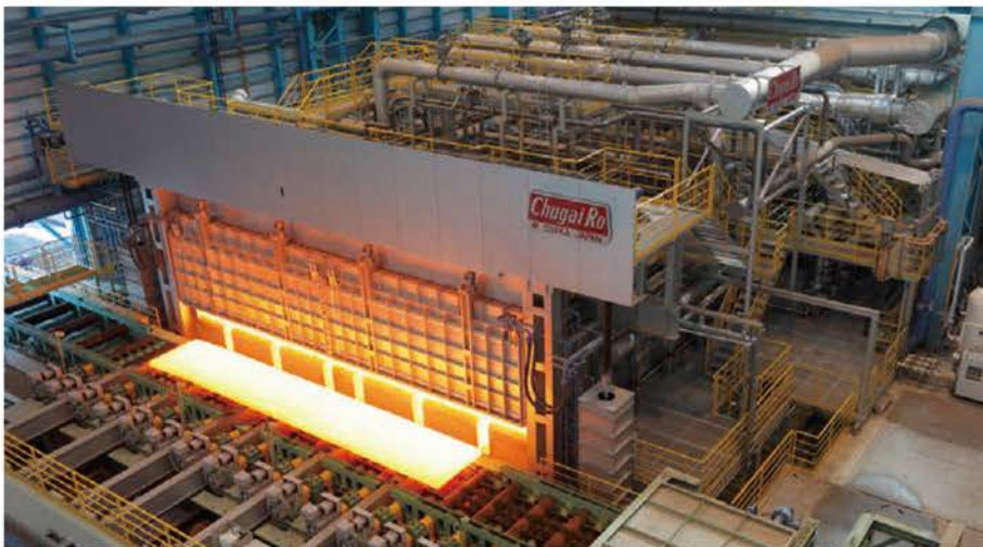
Walking Beam Type Slab Reheating Furnace 步进式钢片加热炉
