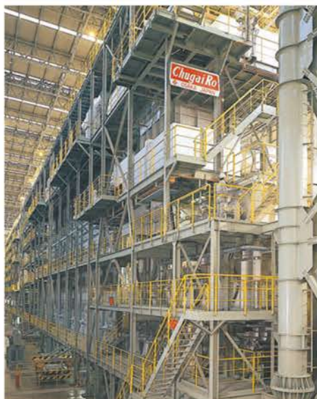
Continuous Annealing Line for Cold Rolled Steel Strip (CAL) 冷轧钢板连续退火炉 (CAL)
